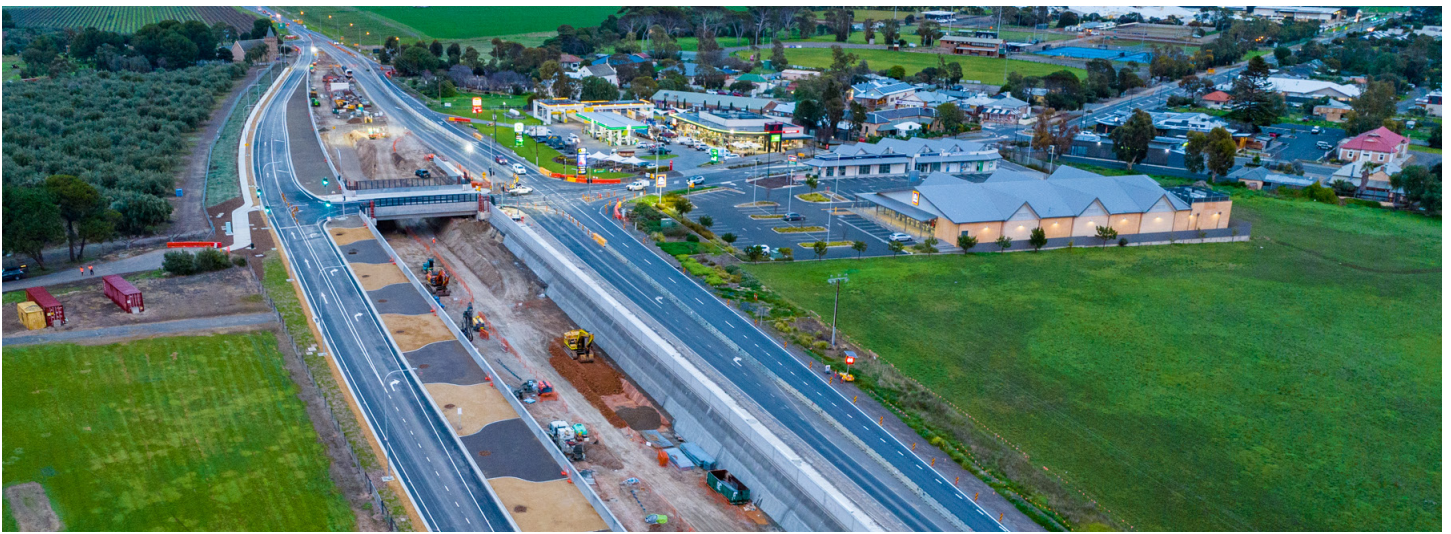
Image: Looking south along Main South Road as traffic moves over the new surface level bridge at Port Road, Aldinga 18 July 2023
